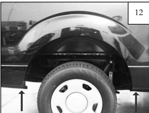
Remove two factory bolts with a 10mm socket wrench. (Note: New hardware is being supplied see Step 17)
