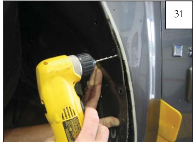
With 3/32" drill bit, drill through mark and the bent tabs of metal behind them for three locations along edge of wheel well.
