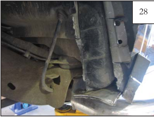
Cut pinch seam at mark made in previous step. Bend flange back even with firewall.
