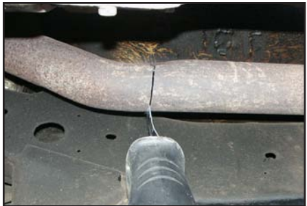
Cut after the bend of the downpipe
