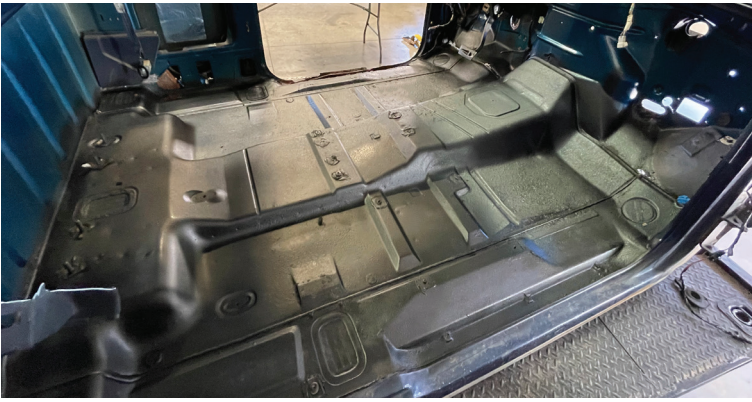
FIG. 1 Remove seats, console & carpet. Clean dirt/debris and recommend using sealer on any rust spots (View from passenger side)
