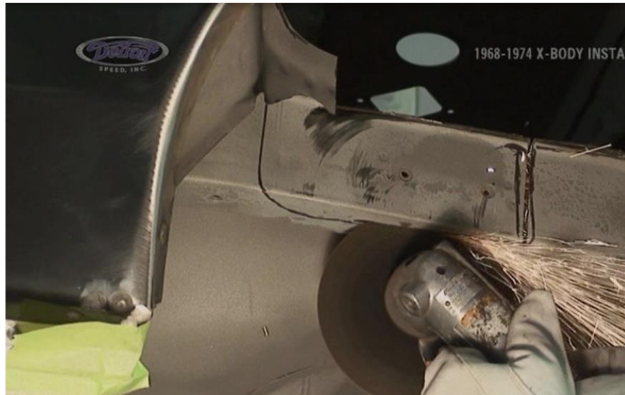
Figure 35 - Passenger Side Framerrail
