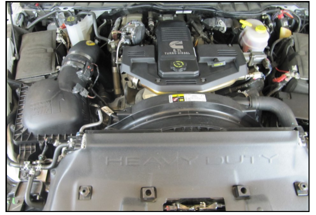
11. Double check your work. Make sure all Clamps are tight and reconnect the negative battery cables.
