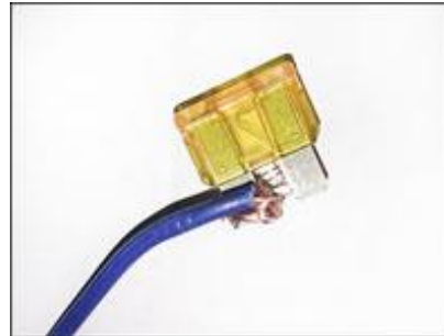
Wire Jammed Into a Fuse
