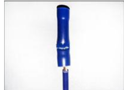
Broken Butt Connectors
