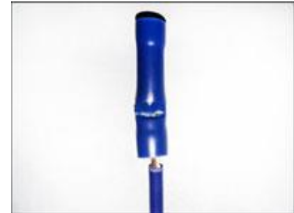
Broken Butt Connectors
