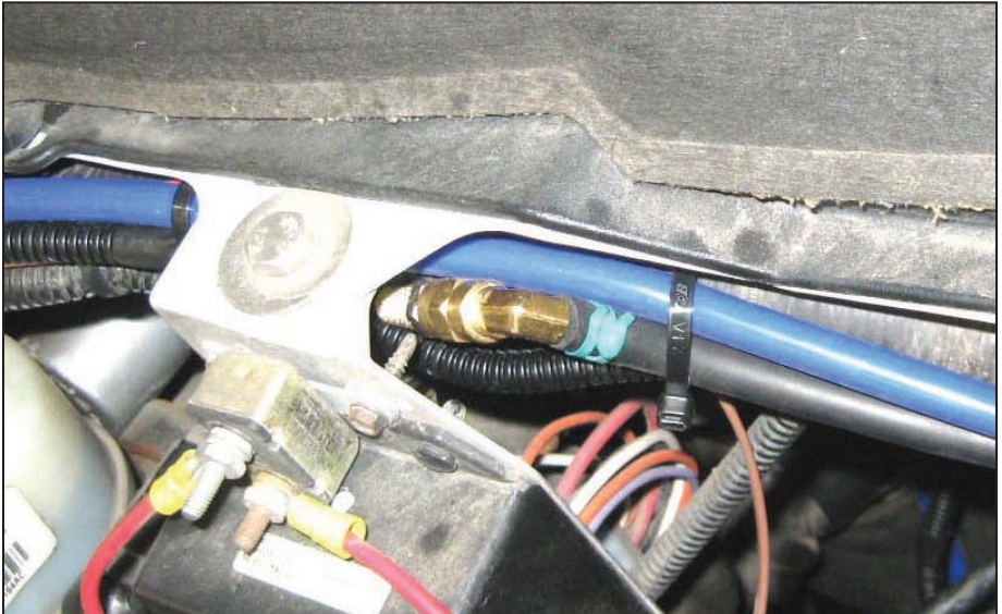
Figure 19 Vent Line with Breather Assembly, Left Side Engine Compartment
