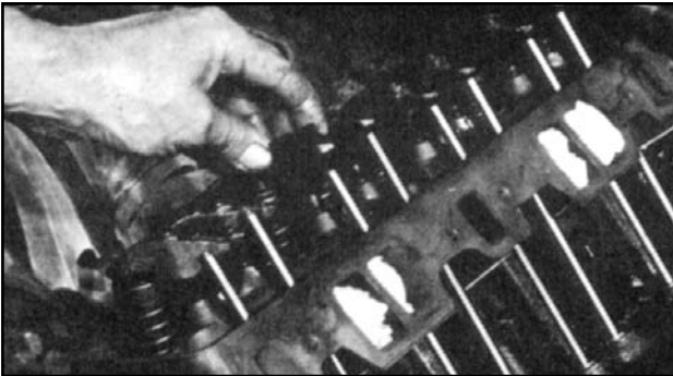
Figure 9. Install the rocker arms carefully, making sure that everything is in place and seated properly. Run the adjusting nuts down just enough to keep everything in place. DO NOT TIGHTEN THEM BEFORE ADJUSTING THE VALVES!
