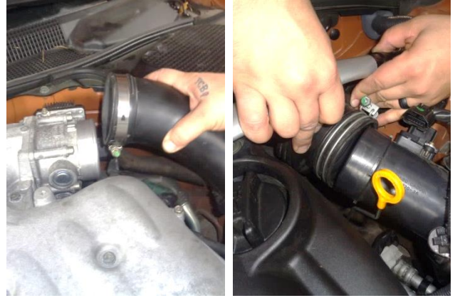
10. Separate the duct from the throttle body and the airbox, then carefully roll the duct slightly away from the engine.
