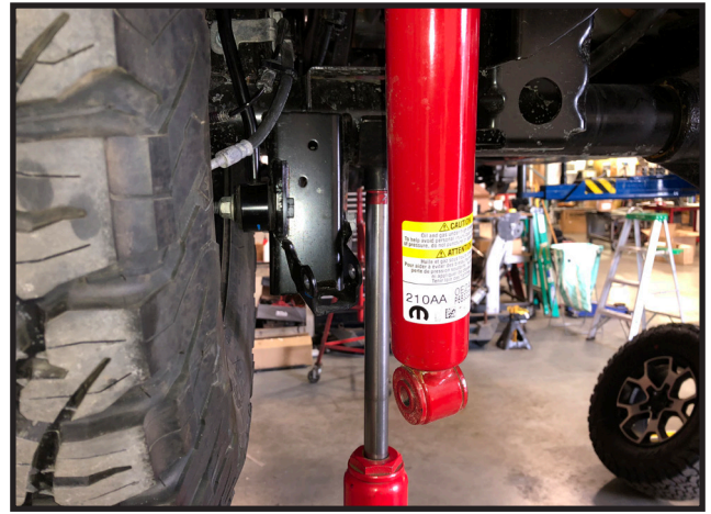
22. On both sides, remove the lower mounting hardware for the sway bar endlinks. Save the hardware.
