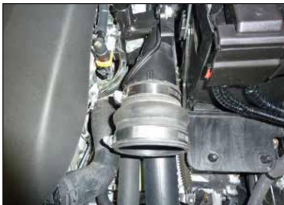
16. Install the hump coupler (5-574) onto the turbo inlet pipe and secure with the provided hose clamp.
