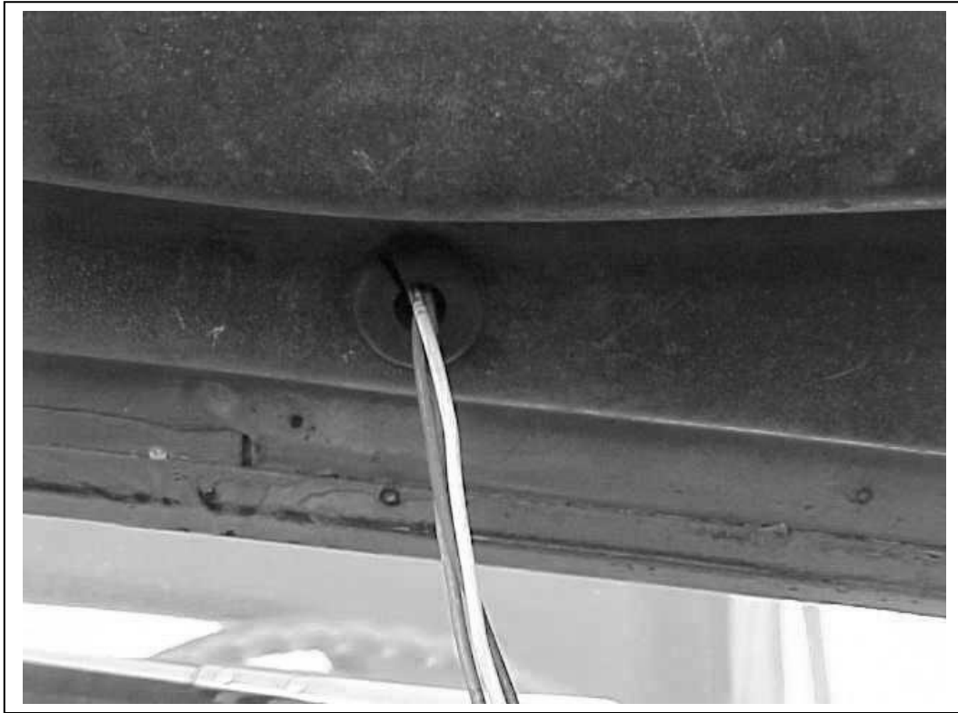
Figure 7.10 Hood Section Wiring (Routed through the bottom of the hood and grommet installed.)
