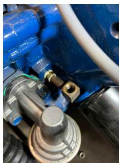
1/4" NPT extension pipe with 90 degree fitting installed.
