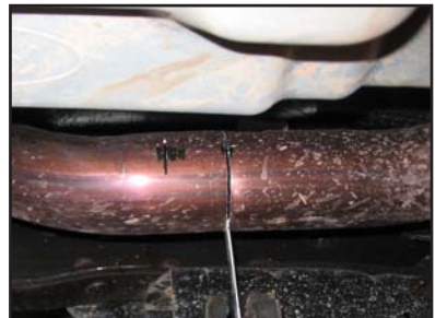
#4 Cut at Bottom of Down Pipe
