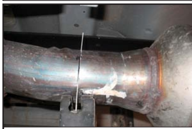
#3 Cut in front of Catalytic Converter
