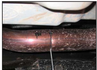
#4 Cut at Bottom of Down Pipe
