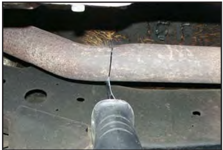
Cut after the bend of the downpipe
