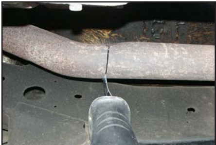
Cut after the bend of the downpipe
