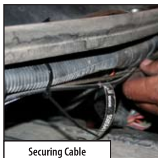
Pyro Probe Installed
