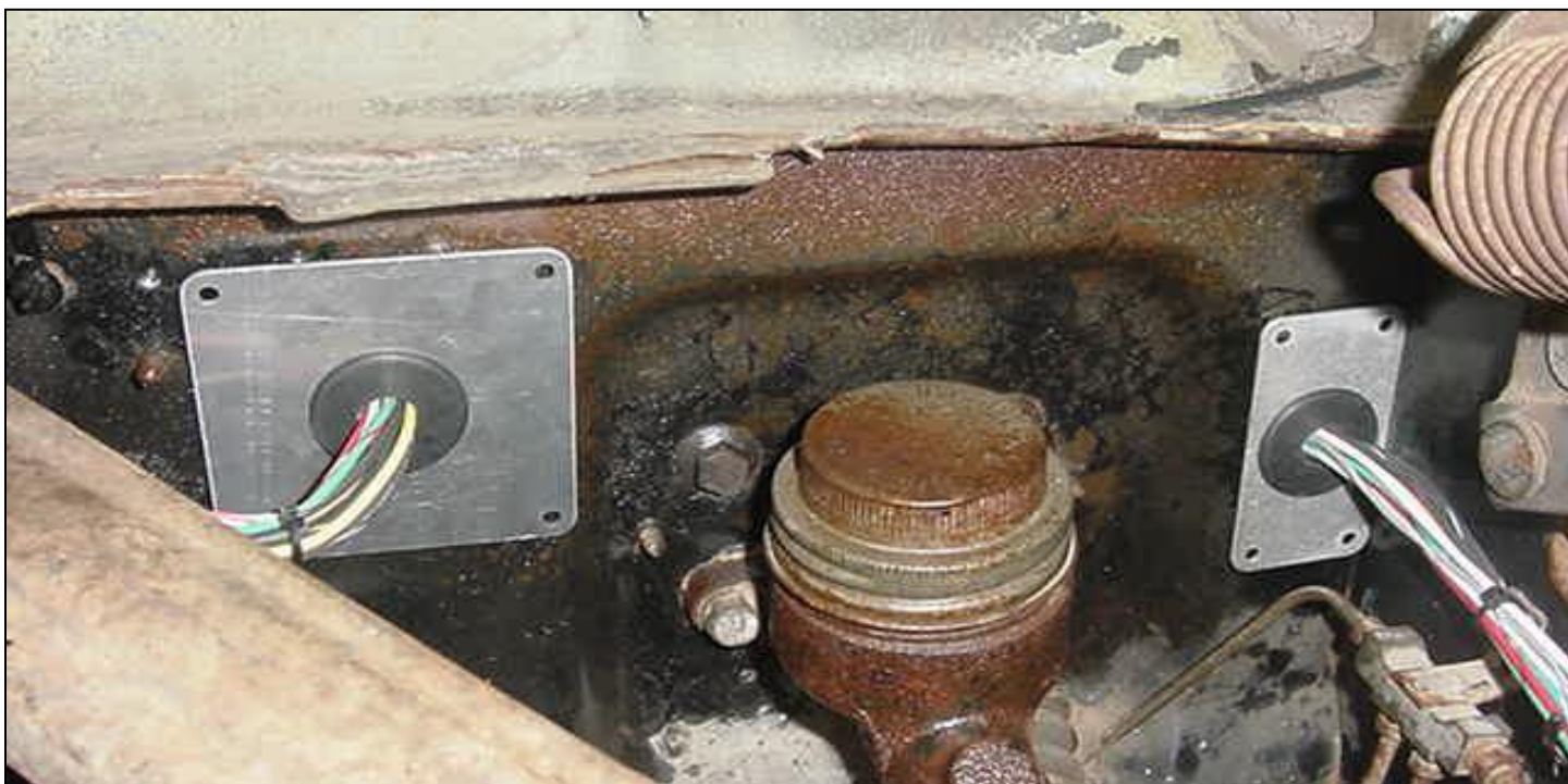
Figure 4 Pass Through Plates and Grommets
