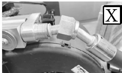
Improperly Seated O-ring Land
