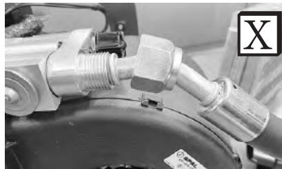
Improperly Seated O-ring Land
