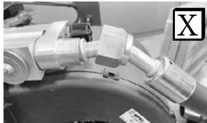
Improperly Seated O-ring Land
