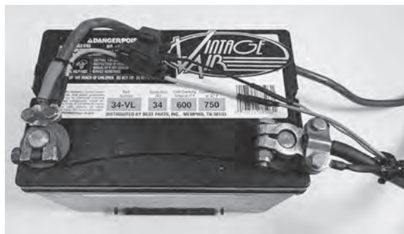
Completed Installation Shown
