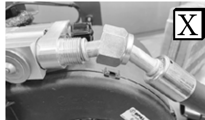
Improperly Seated O-ring Land
