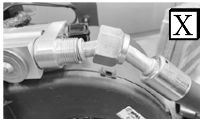
Improperly Seated O-ring Land
