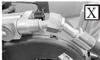
Improperly Seated O-ring Land
